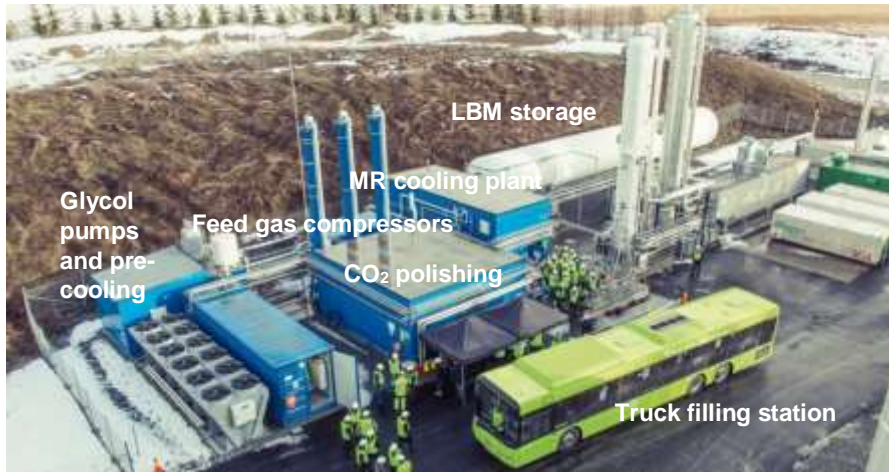
Figure 8. The EGE biogas liquefaction plant (modified from Sherrard 2014).
